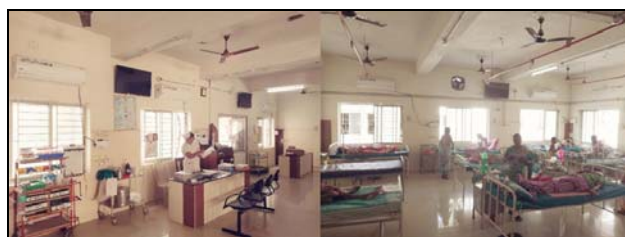
Fig 5: Air conditioner units and LED televisions installed in post-operative ward.
